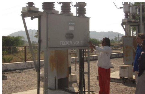
Inspection of Potential Pilot Project Feeders
